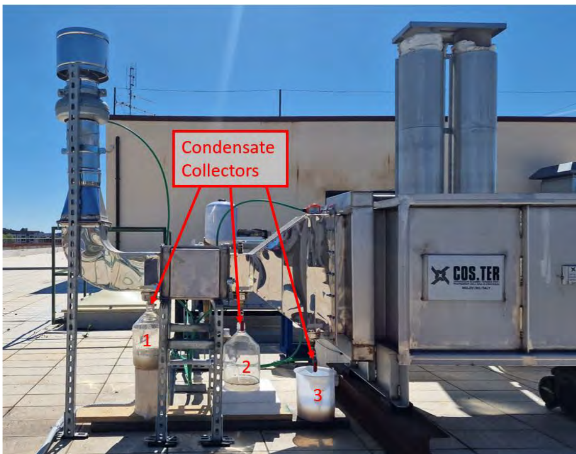
Figure 6. Condensing draining points.
